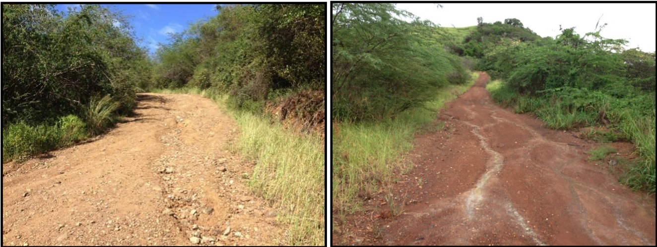
Figure 18. Dirt roads as a source of sediment (note the surface runoff over the roads creating erosion and resulting in fine sediment losses)
