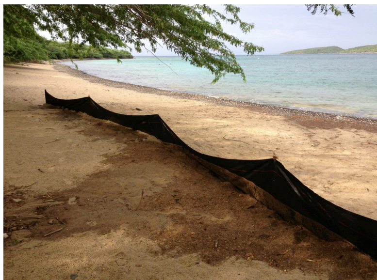
Figure 21. Silt fence at the Tamarindo restoration holding back sediment from nearshore waters from an upland dirt parking lot and restoration project
